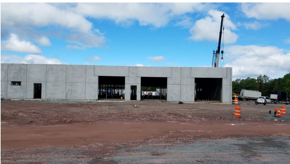
Walls are up and cells are coming for the new Sullivan County Jail in Monticello.
